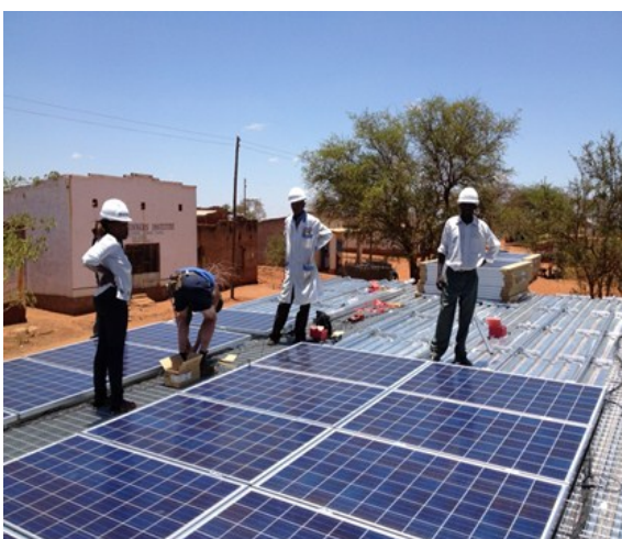
E4D project's solar panels fitted on a canopy
